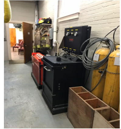
Figure 46 Compressed Air Cylinders in Apparatus Bays
