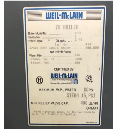
Figure 58 Well-McLain Boiler Plate
