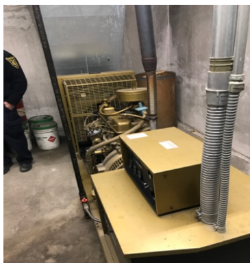
Figure 59 Emergency Standby Generator Basement Level
